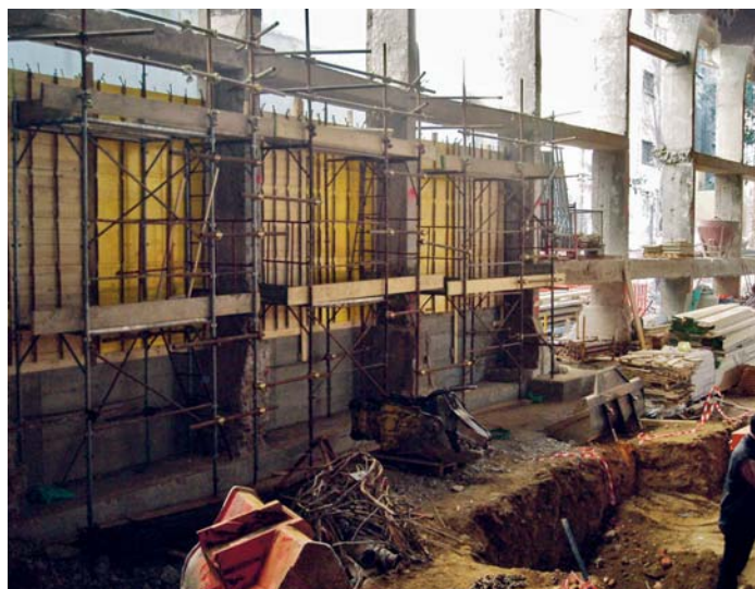
Soil retaining walls made with structural CALCESTRUZZO FIBRATO for the reconstruction of a commercial area in Milan.
